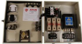
ACH DOL Three Phase Control Panel Board
